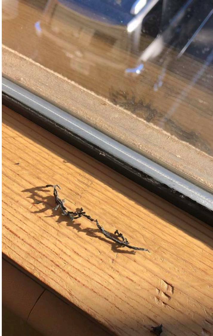
Asbestos containing window caulk
