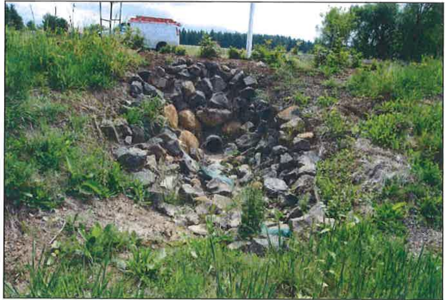
Photo B3. New culvert outlet upstream of the Lucini property. This view looks east toward Boones Ferry Road.
