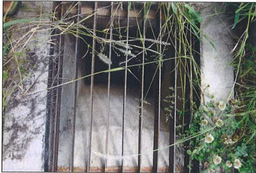
Photo B1. New Stormwater Inlet #1 (North).
