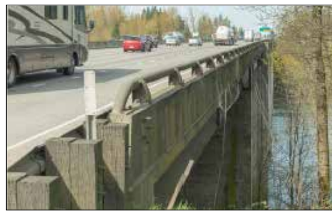
As this southbound view demonstrates, there is little protection for bicyclists and pedestrians to safely cross the I-5 Boone Bridge.
