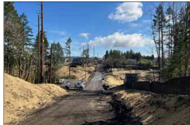
Crews have been preparing Boeckman Road for a project to bridge over the Boeckman Dip.
