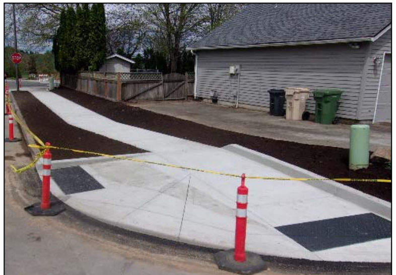
New sidewalk between Jamaica and Wilsonville Road across from Graham Oaks Nature Park.
