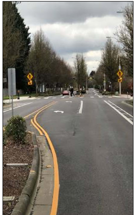
Repaved and restriped roadway, the replaced curb ramps (which now meet ADA standards), as well as the new pedestrian activated beacons on Wilsonville Road at Guiss Way/ Orchard Drive
