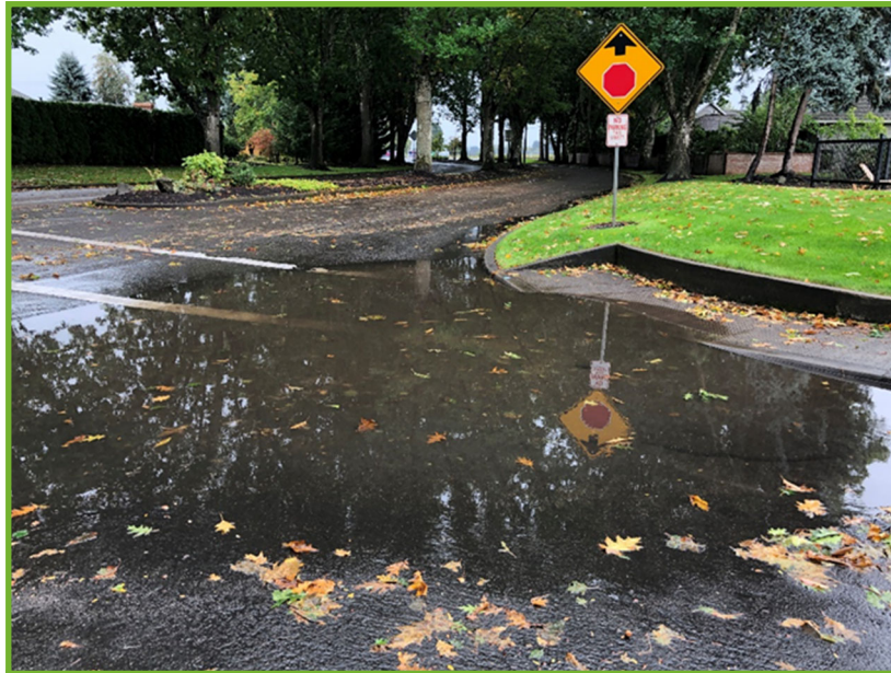
Standing water after heavy rain
