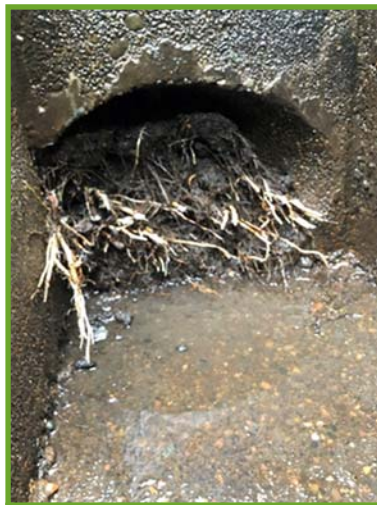
Roots in a catch basin
