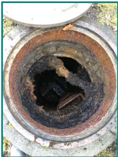
Left: Root intrusion in an old manhole.
