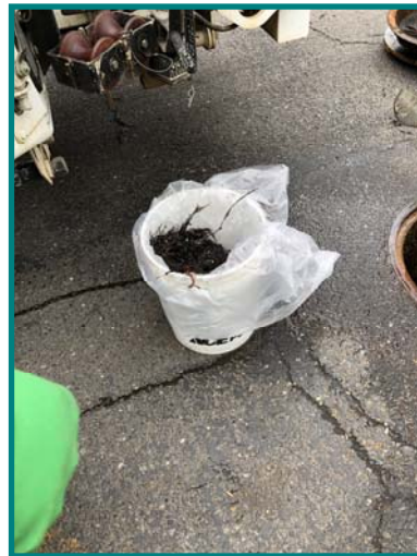
Left: Roots removed from sewer manhole.
