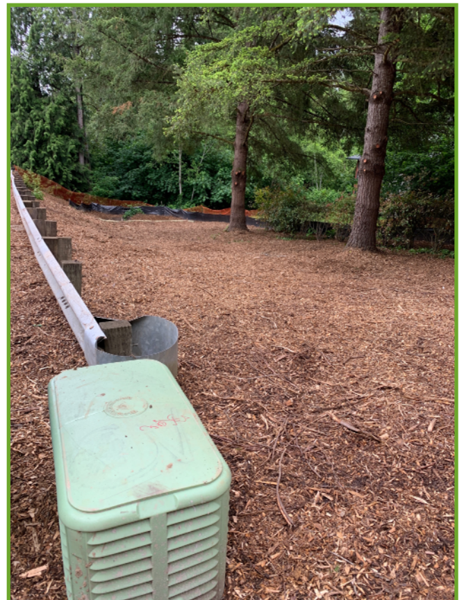
Looking west towards Boeckman Creek with the temporary erosion control measures in place.
