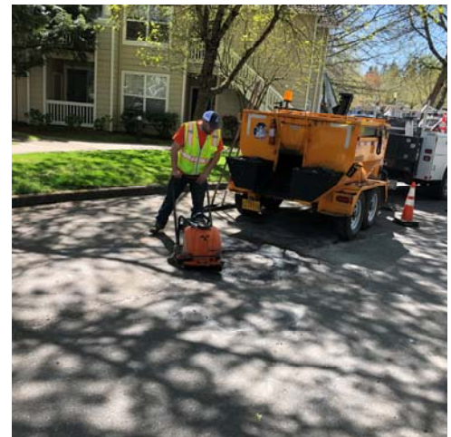
Asphalt patch around casing ring
