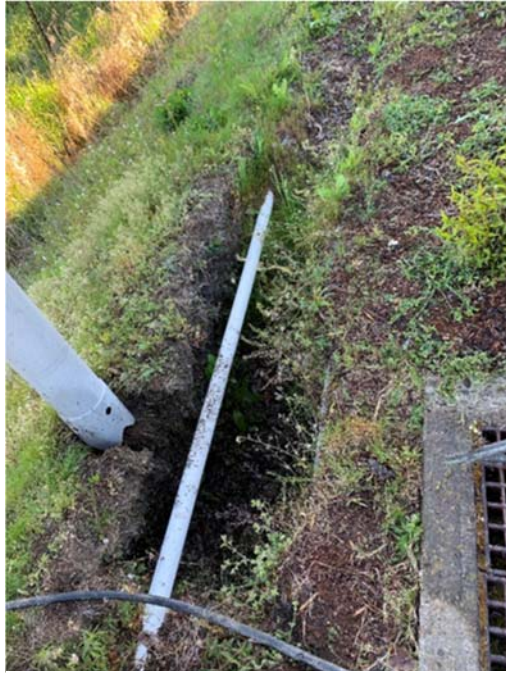
Sink hole along Boeckman Road
