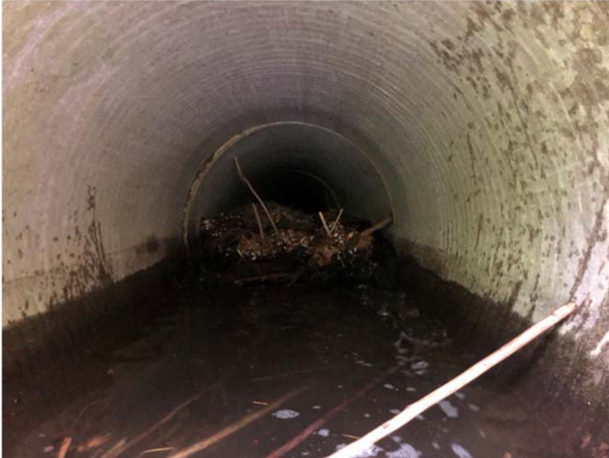
Beaver's dam inside a stormwater pipe
