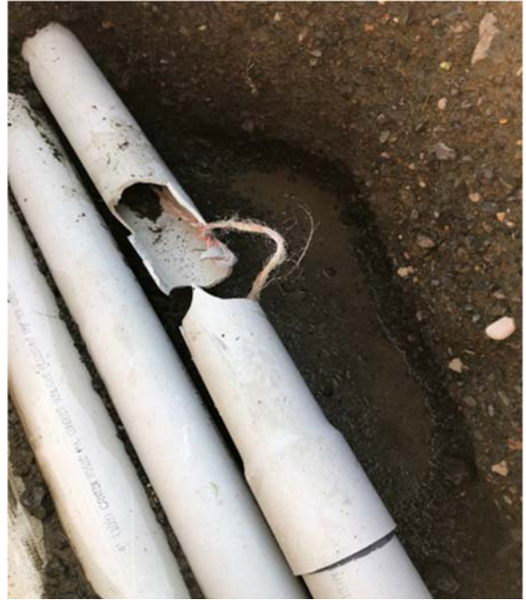
Broken, empty pipe caused water erosion which created the sink hole
